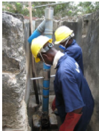
Figure 2: Emptying of Faecal Sludge
