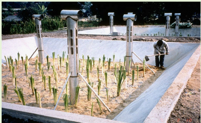
Photo 9: New installation of a constructed wetland with ventilation pipes at the Asian Institute of Technology (AIT) in Bangkok, Thailand. (Sandec, 1997)
