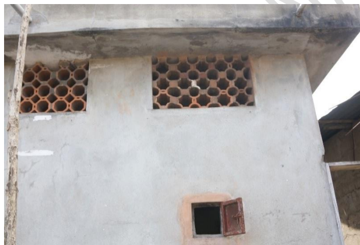
Photo: PATH Figure 6. A small window with a latching door enables vidange trucks easy access to tanks for emptying.
