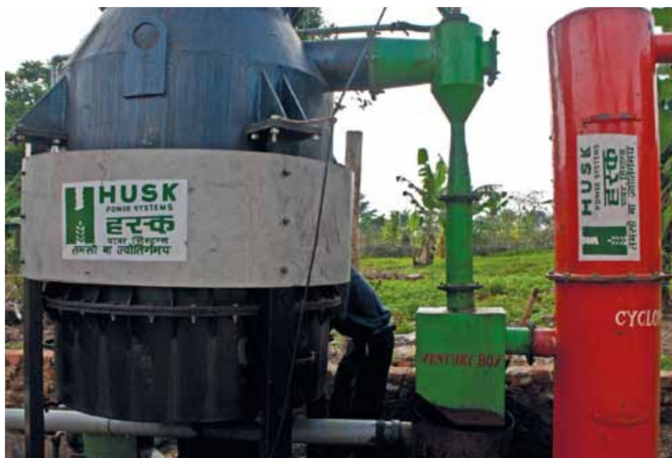
Figure 10.12 Iiribogo gasification project utilising corn husks and sawdust, located in Muduuma Sub-county, Mpigi District, Uganda (photo: Linda Strande).
