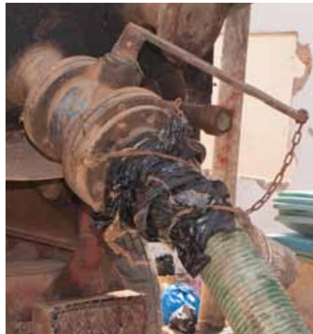
Figure 4.13 Example of an improperly maintained hose held together with plastic bags and twine (photo: David M. Robbins).
