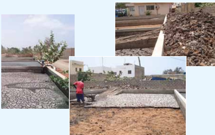
Figure 7.6 Unplanted drying beds, sludge removal and accumulation at Cambérène treatment plant, Dakar, Senegal (photos: Pierre-Henri Dodane).
