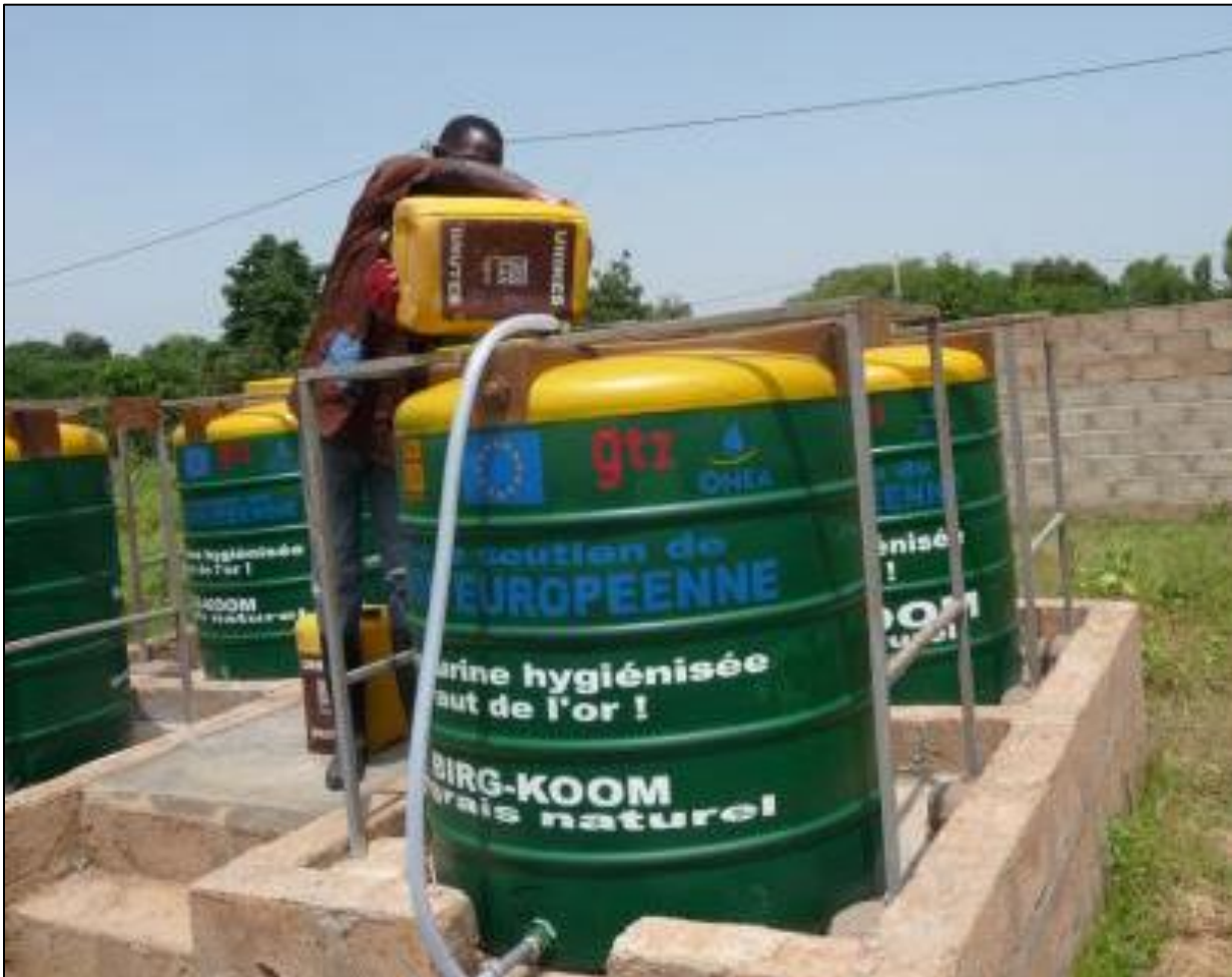
Urine collection in Burkina Faso (Credit: Sustainable Sanitation Alliance)
