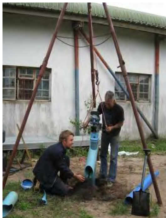
Figure 4.9. Using a tripod to support the Pit Sludge Auger while it is manoeuvred around the sludge
