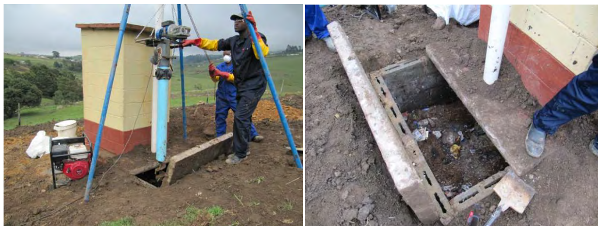
Figure 4.11 Using the auger to empty a VIP pit (left). The amount of rubbish which the pit contained (right) made it impossible for the auger to remove sludge.
