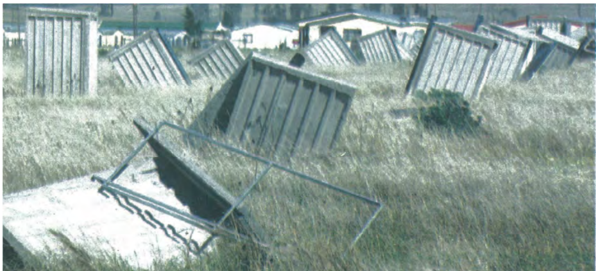
Figure 7.2 Precast VIPs erected at Dutywa in the Eastern Cape which have collapsed due to inadequate foundation preparation
