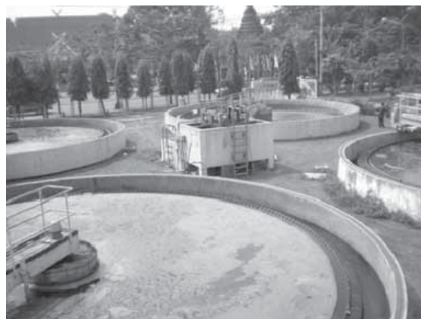
Photo 2 Chiang Mai University Wastewater Treatment Plant (WWTP)
