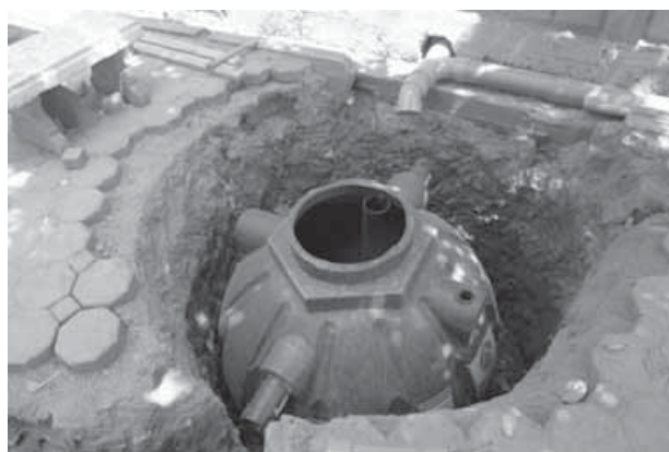
Photo 7 On-site treatment system for both black and gray water being installed in Chiang Mai University campus
