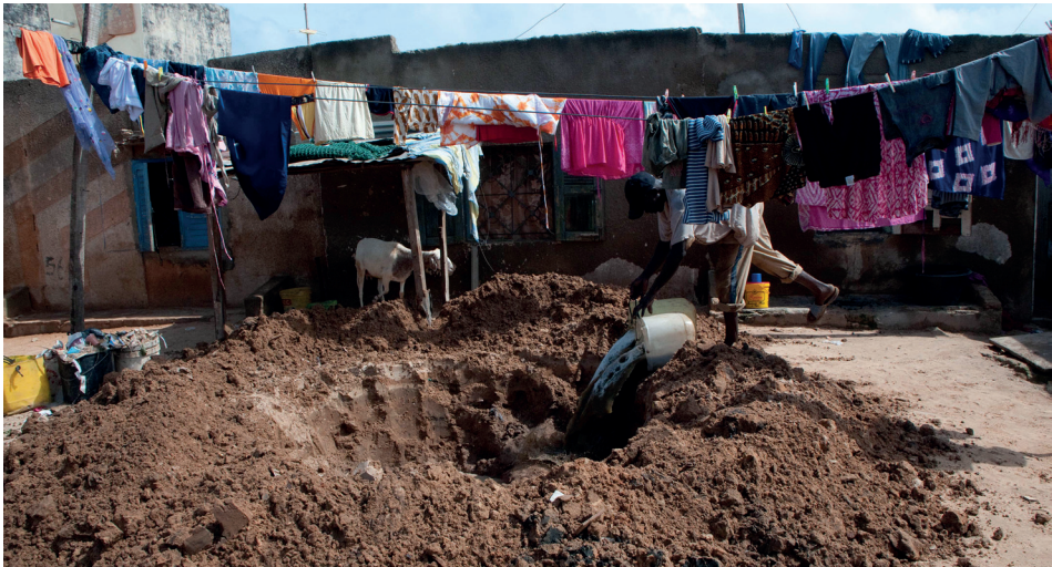
Figure 14.9 Faecal sludge manual emptying and burying within the courtyard (photo: Linda Strande).
