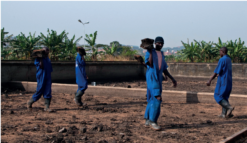
Figure 11.7 Sludge removal from drying beds at the Bugolobi Treatment Plant in Kampala, Uganda (photo: Linda Strande).
