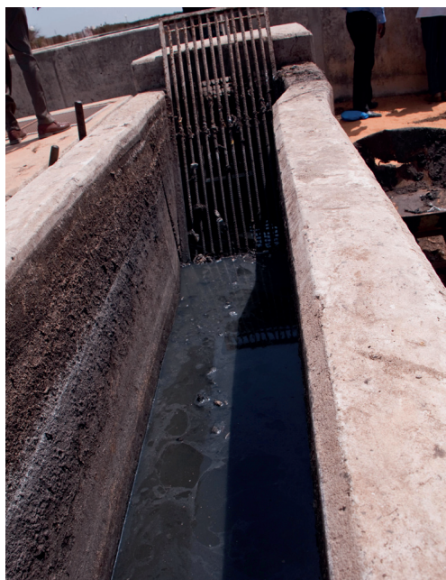
Figure 8.5 A holding -mixing tank with a bar screen is used in Senegal to prevent garbage from clogging the bed (photo: Linda Strande).
