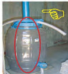
PIPE TOO SHORT (SHOULD END ABOUT 3" ABOVE BOTTOM)
