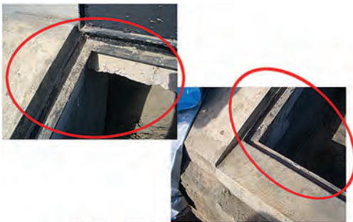
POOR DESIGN OF SLOPING COVER ALLOWING RAINWATER TO ENTER PROCESSING CHAMBERS
