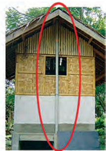
DIAMETER TOO SMALL
