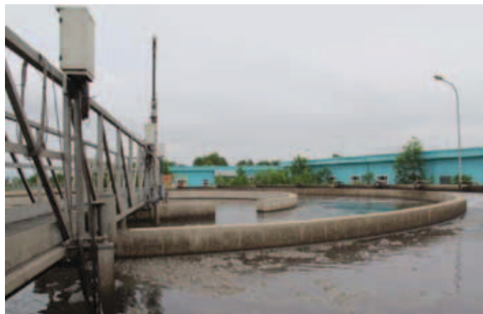
Figure 2.3 Bac Giang Wastewater Treatment Plant
