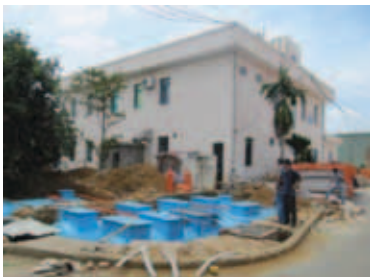
Decentralized wastewater treatment plant in Phu Cat, Hoa Lac, Hanoi suburb
