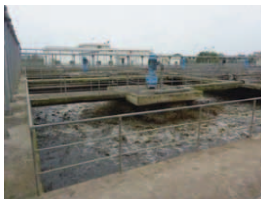
Figure 3.4 Activated sludge WWTP
