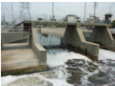
Diluted incoming flow from open canal of CSS is not suitable for invested hi-tech SBR treatment plant (6)
