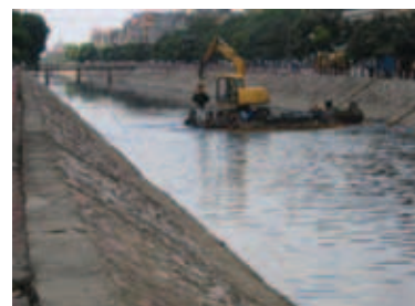
Treatment and disposal of dredged sludge are issues
