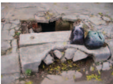
Street manholes are not always maintained
