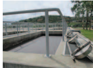
Scum collector at Imhoff tank invented by Mr. Khai, Da Lat WSS Co.
