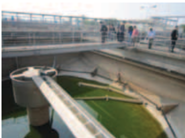
BTL WWTP (Hanoi city) is under-utilized due to lack of sewer connections
