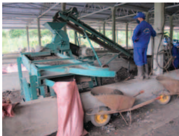
Figure C17: Making Compost From Sludge at the Da Lat WWTP
