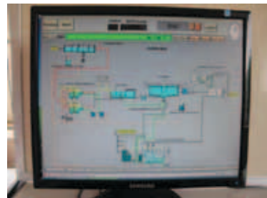
Hi-tech SCADA system does not operate in Bac Giang WWT
