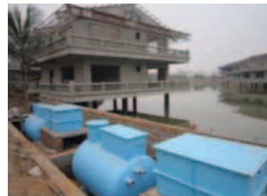
Packaged w/w treatment systems for Eco-resort in Dong Anh district, Hanoi suburb
