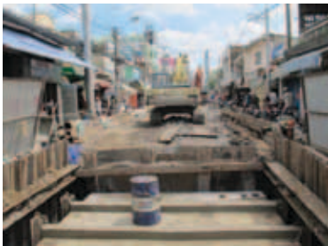
Installation of sewers in existing urban areas is always a challenging task
