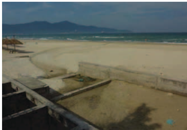
Figure 3.3 Discharge of CSS Overflow to Da Nang Beach
