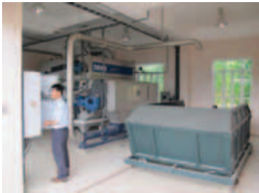
“Unused” sludge drying machine in 2-year- operation Bac Giang WWTP
