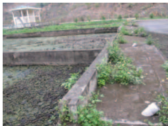
Figure C14: Sludge drying bed with non-functioning FS receiving building in the background
