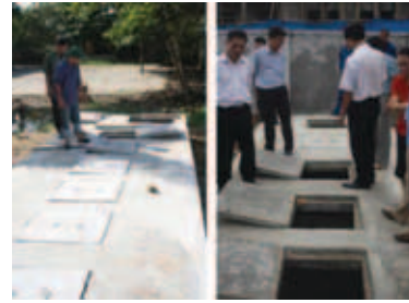
Decentralized wastewater treatment plant for School in Vinh City (7)
