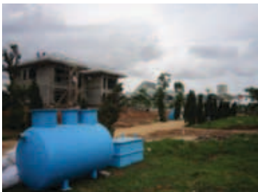
Packaged w/w treatment systems for villas at the National Congress Centre, Hanoi
