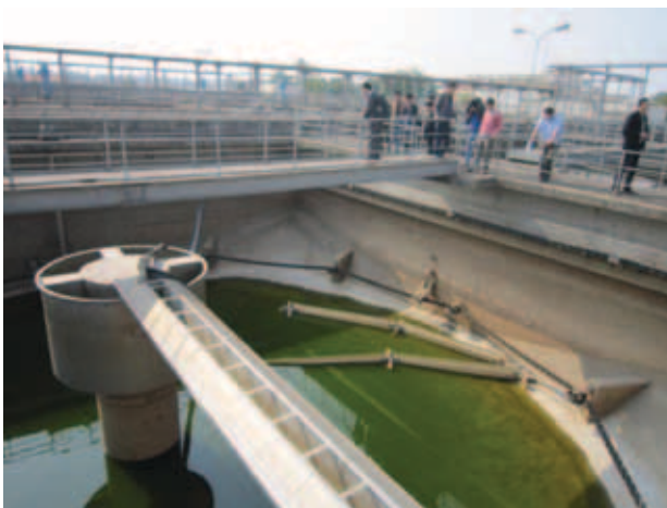
Figure C15: The WWTP in Hanoi city under-utilized due to lack of sewer connections
