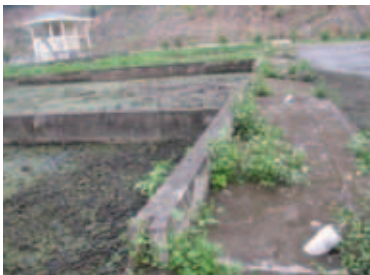
Sludge drying bed at Bai Chay WWTP.
