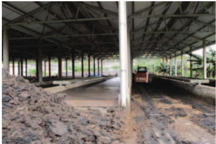
Figure 1.7 Sludge Drying Bed at Da Lat WWTP
