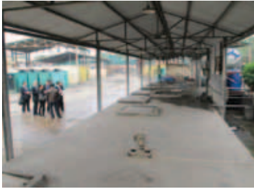
Septage holding and thickening is a major treatment step in Cau Dzien waste treatment station, Hanoi
