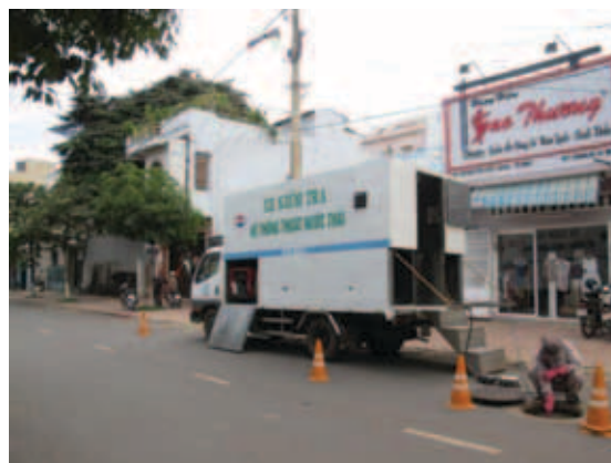
Figure C18: Inspection of Separate Sewer System Network with CCTV in Buon Ma Thuot City
