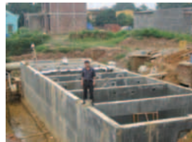
Baffled septic tank for a new development area, Xuan Mai town, Hanoi
