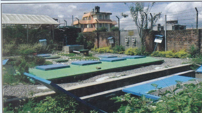
Lubu Fecal Sludge Treatment Plant
