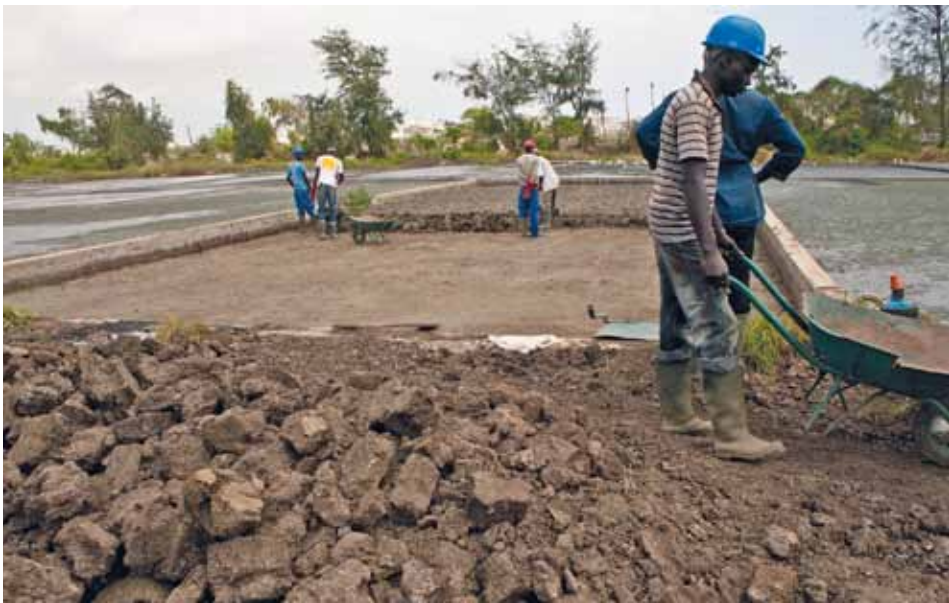
Figure 7.5 Removing sludge from unplanted drying beds at Cambérène treatment plant, Dakar, Senegal (photo: Linda Strande).
