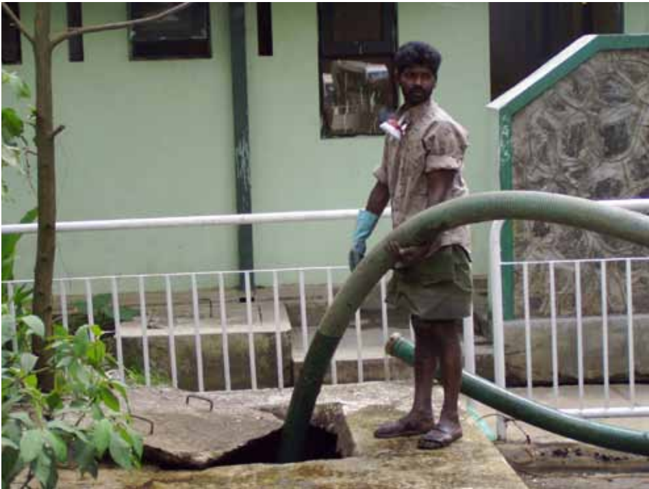
Figure 4.1 Emptying operation of faecal sludge from a septic tank using vacuum equipment. Job safety would be improved by better protective equipment (photo: David M. Robbins).
