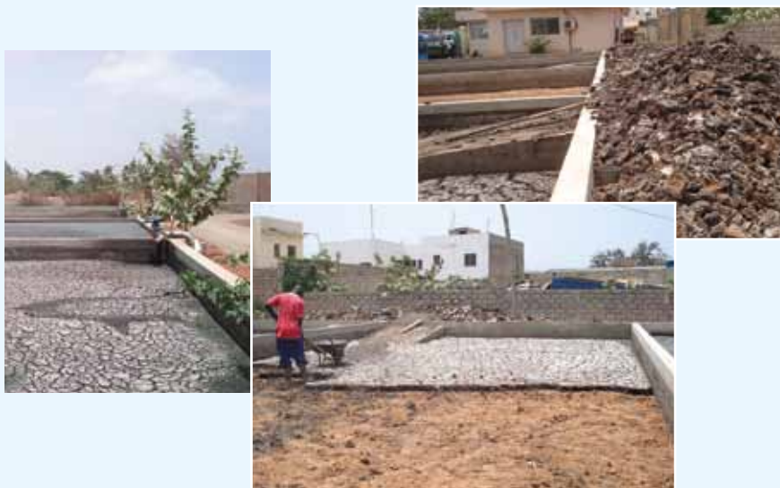
Figure 7.6 Unplanted drying beds, sludge removal and accumulation at Cambérène treatment plant, Dakar, Senegal (photos: Pierre-Henri Dodane).
