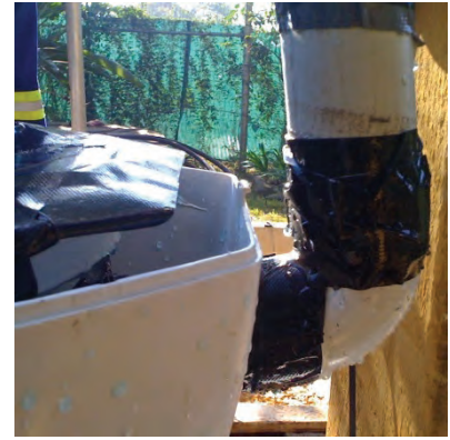
Figure 2.11 U shaped pipe providing inlet to flushing water
