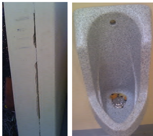
Figure 5.1 Cracking door frames and urinals without flushers reported to eThekweni
