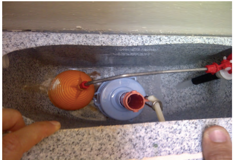
Figure 2.2 A longer arm was needed for the Atlas cistern so that it could be bent down to limit the flush to 2.5 ℓ
