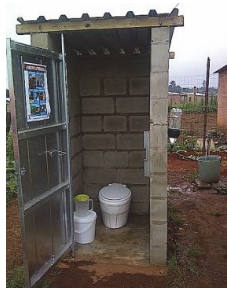
One of the installed pour-flush systems.
