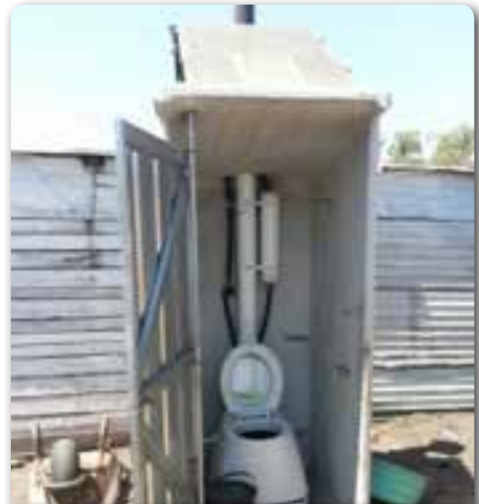
Existing EcoSan Toilets
