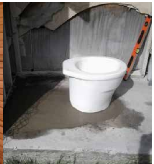
Toilet 3 Installation existing dilapidated structure, (note septic tank was located directly below toilet so toilet had to be set forward to accommodate long P-trap)
