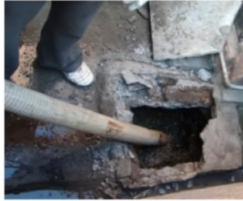
Emptying when the tank is full
