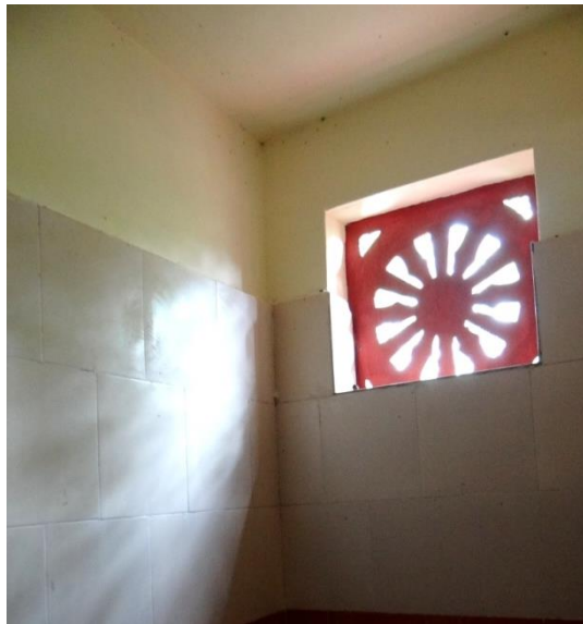
Proper considerations for natural ventilation in newer blocks
