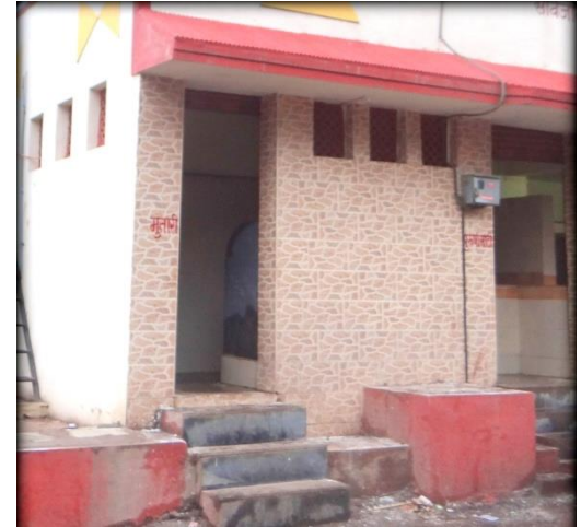
In some cases, urinals are also provided in the blocks
