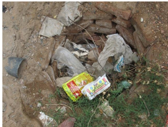
Non - functional leach pit
