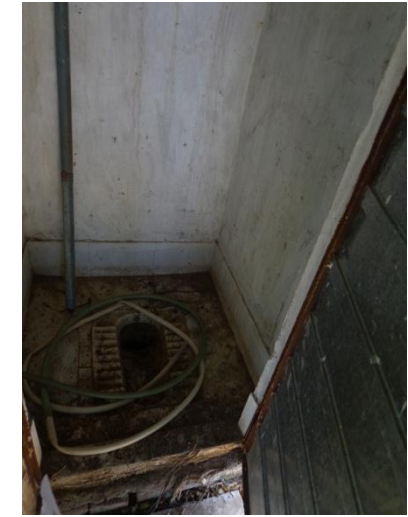
Condition of toilet in Dongal talavadi
