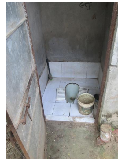
Condition of toilet in Khajur talavadi
