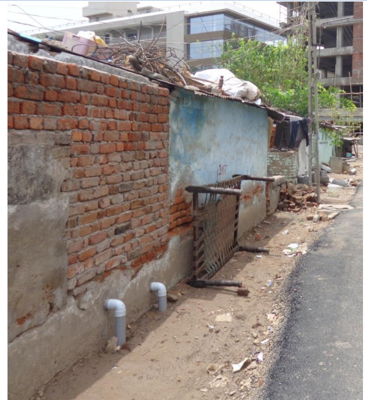
Toilet connected with sewerage system
