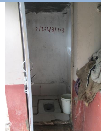
Toilet with Single pit system
