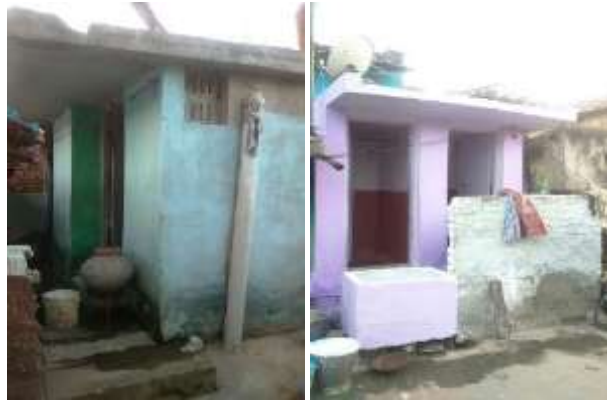
IHHL & Septic Tanks
