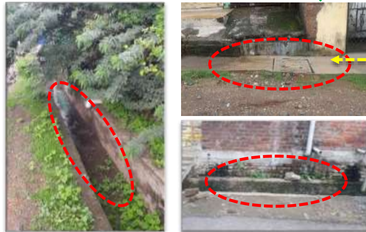
Open and Closed drains
