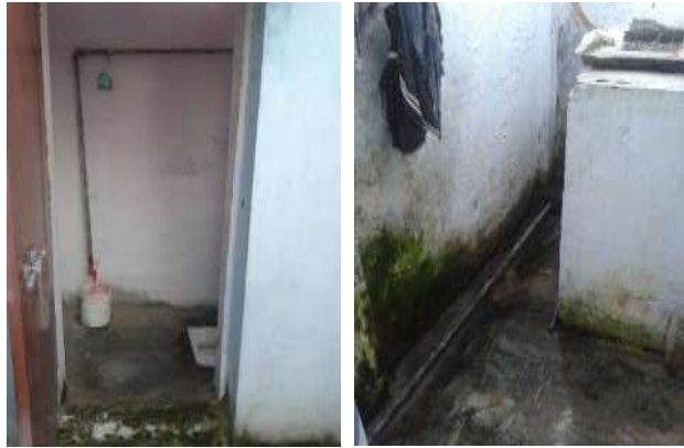
IHHL & Septic Tanks
