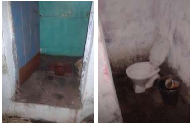
IHHL & Septic Tanks
