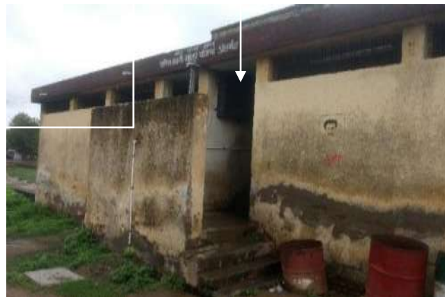
Community toilet (10 seats) at Compact STP
