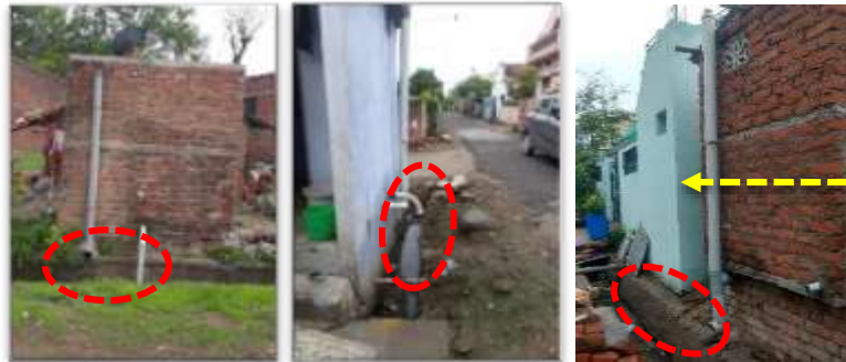
HHs waste water into open drains
