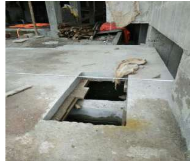
Oversized septic tank in bungalow
