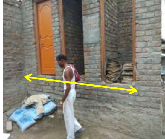
Septic tanks are below the toilets and don't have access
