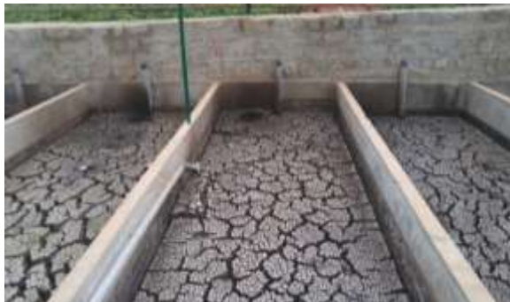
Sludge drying bed
