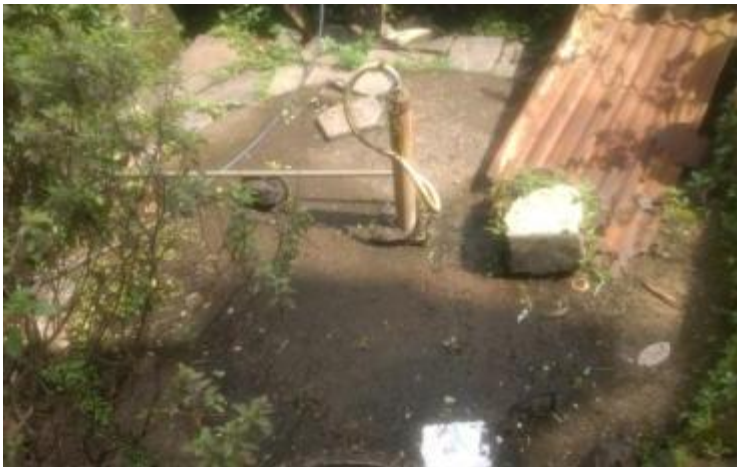
2. A 2-storied bungalow here has built a circular septic tank of 8 ft diameter 15 years ago. It is cleaned every 5-6 years.
