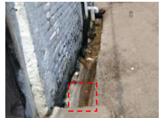
Some insanitary toilets found in slums
