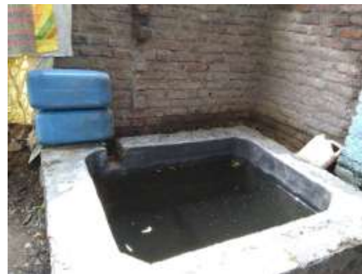
Few septic tanks without chambers
