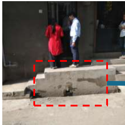
Over flow of septic tanks and kitchen enters the road side drains
