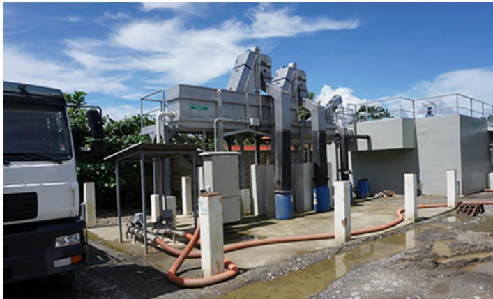
Figure 3. EnviroKonsult septage treatment plant using screw press and sequencing batch reactor technology
