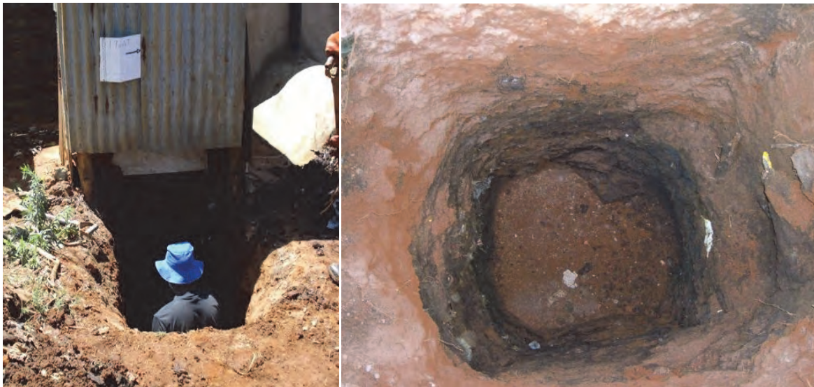
Figure 3.1 Manual excavation of a pit. The start of the sludge layer is clearly visible 1.65m below the surface.
