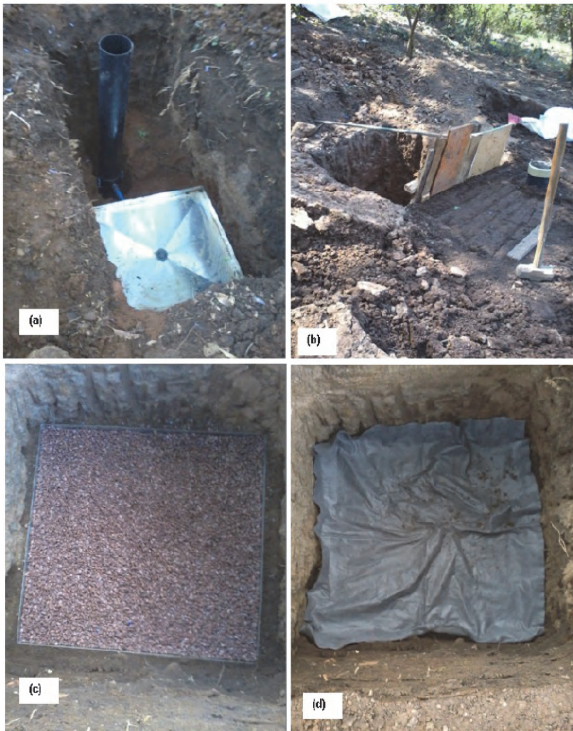
Figure 3.45 Installing pan lysimeter into a pit (a), refilling back the soil (b) and filling 80 mm thick layer of gravel (10 mm dia.) into a pan of 1m wide by 1m long, and a bidim covering the gravel layer (d) to facilitate drainage and prevent soil sediment from entering a drainage system.
