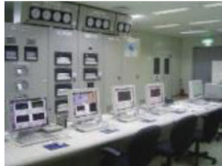
Figure B1.1-3 Central Control Room
