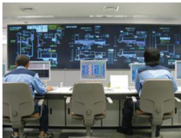
Figure B1.1-4 Main Monitoring Room in Water Reclamation Centre
