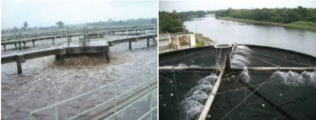
Figure 8.5 Aeration tank (left) and Attached growth system (right)
