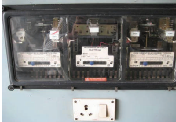
Figure 6.2 Electromagnetic Protective relay
