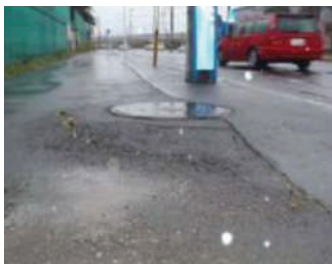
Figure 2.40 Not coinciding with height of road surface
