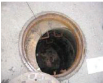
Figure 2.39 Offset of manhole block
