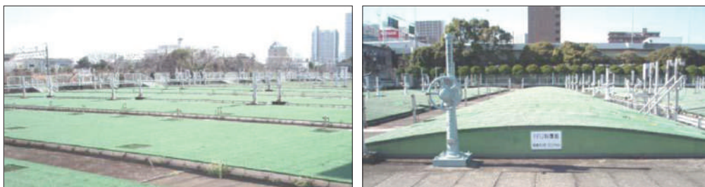
(A) Figure A5.1-1 Covers over sewage structure — Flat type and Dome type (Yokohama City)
