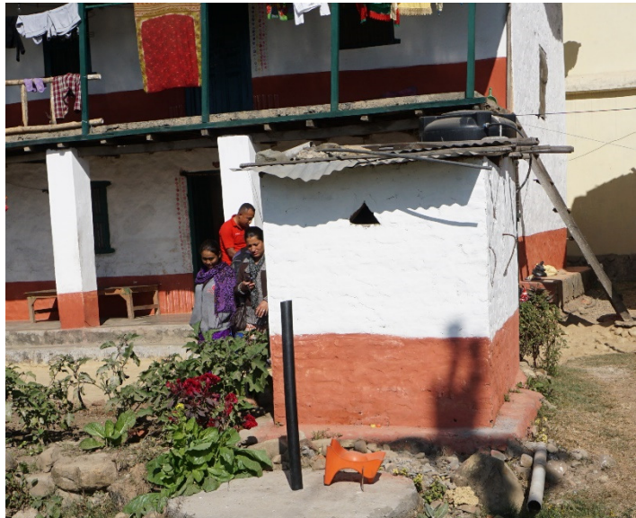
Figure 2. Typical containment tank (off-set pit latrine) of approximately 8 cubic meters in total volume. Notice the vent pipe, which should be extended above roof level for better odor control.
