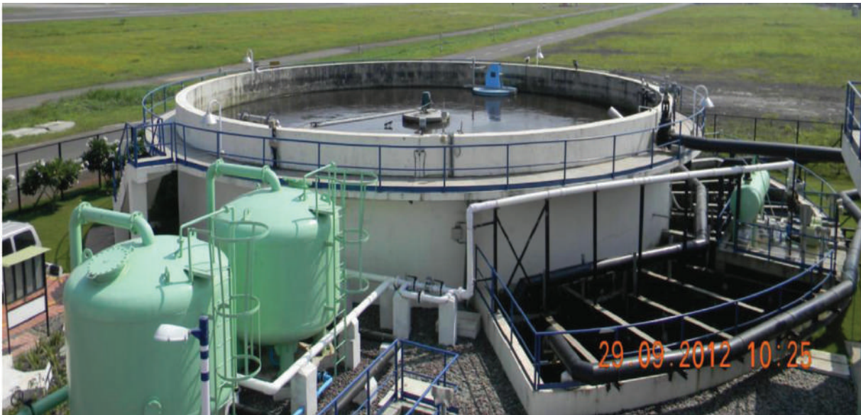
Figure 7.4 Circular SBR based STP at MIAL with floating decanter
