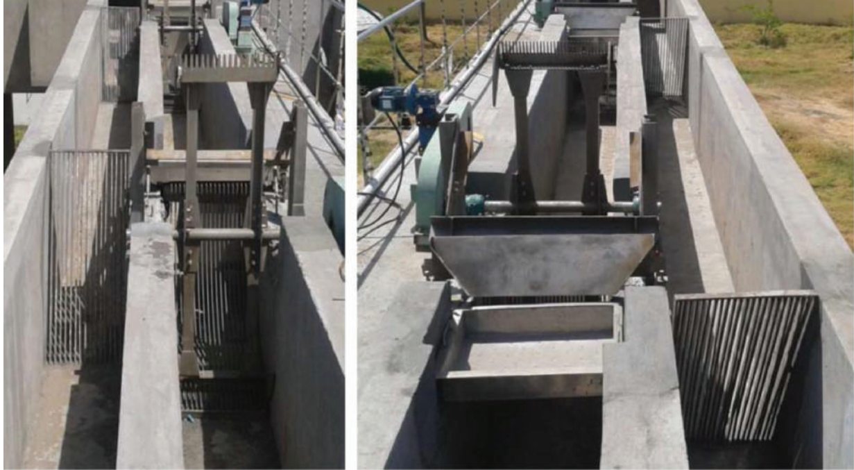
Figure 5.24 UNIDO type circular wedge wire screen seen from upstream at left and from downstream at right in Ramanathapuram STP of Tamilnadu
