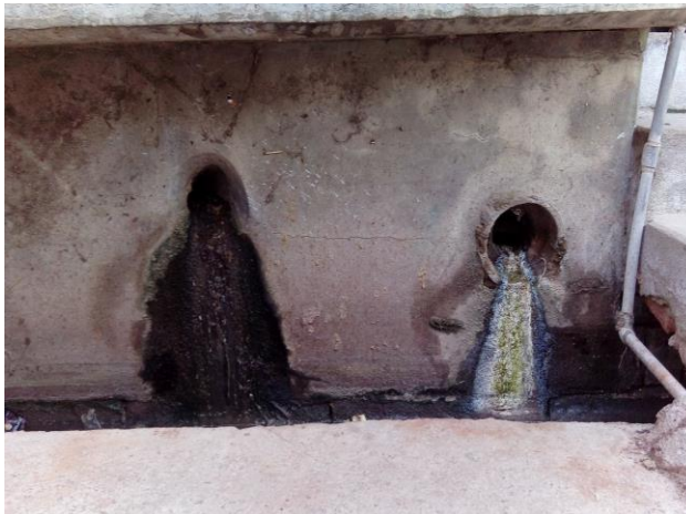
Figure 9: Outlet of a containment unit drains directly into the drains in the street
