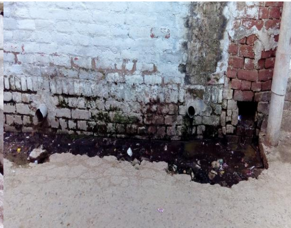
Figure 10: Outlet of a containment unit drains directly into a drain
