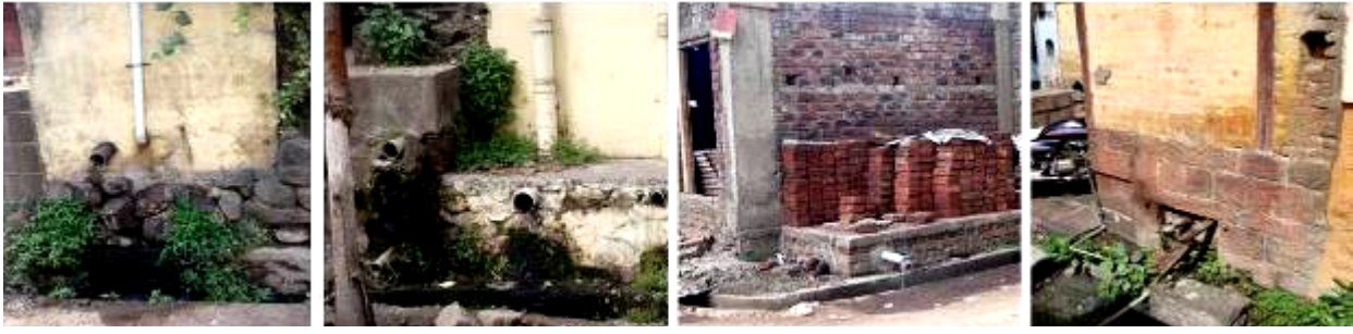
Figure 3: Discharge of black water / effluent from Septic tanks into open drains
