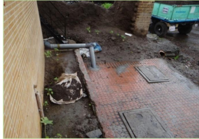
Oversized septic tanks
