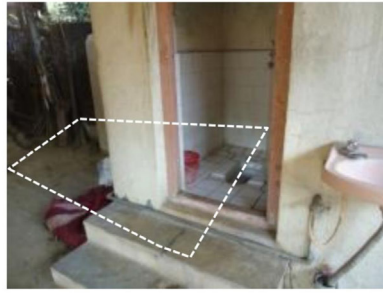
Inaccessible septic tanks with sealed tops
