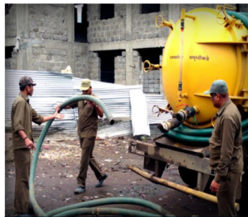
Unsafe handling of septage
