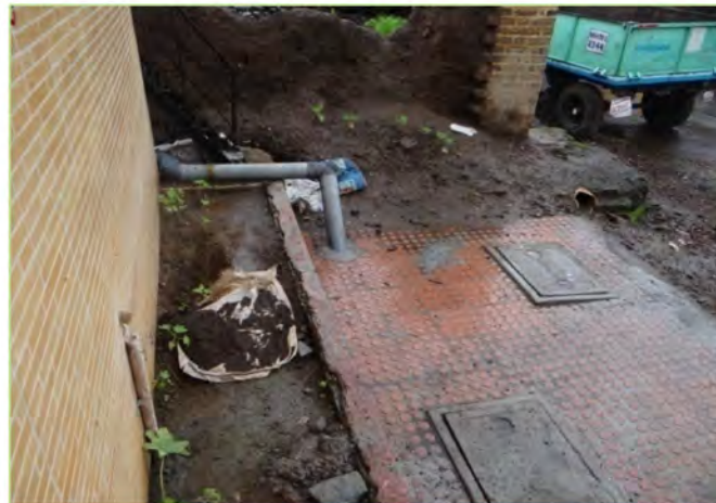
Oversized septic tanks
