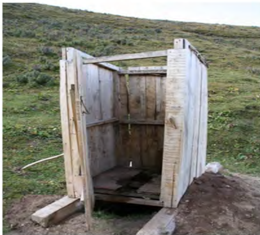
Single pit toilets
