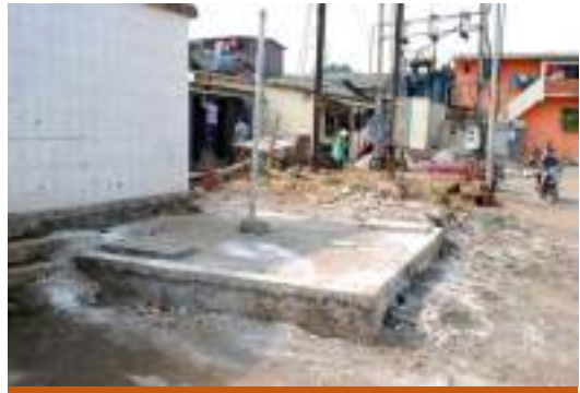
Group septic tanks connected to 25-30 individual toilets in one slum
