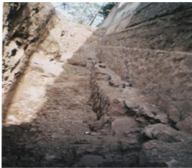
Dilapidated state of water storage tank
