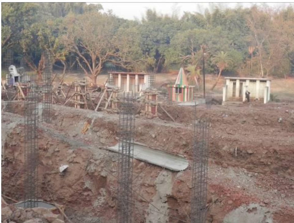
Construction work in progress under the Integrated Housing and Slum Development Programme.
