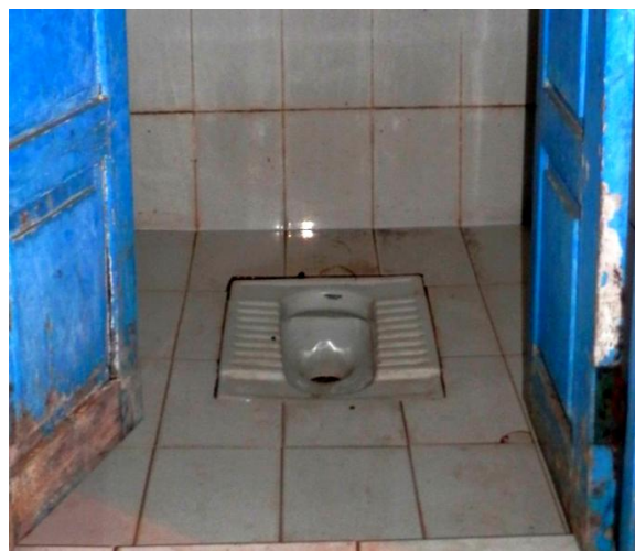
The toilets are reasonably well maintained.
