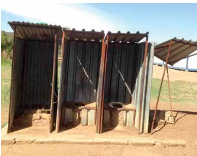
Toilets with missing doors offer learners no privacy when using the toilet.
