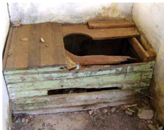
Broken pedestals over pit toilets cause dangerous conditions for learners, especially those in primary school.
