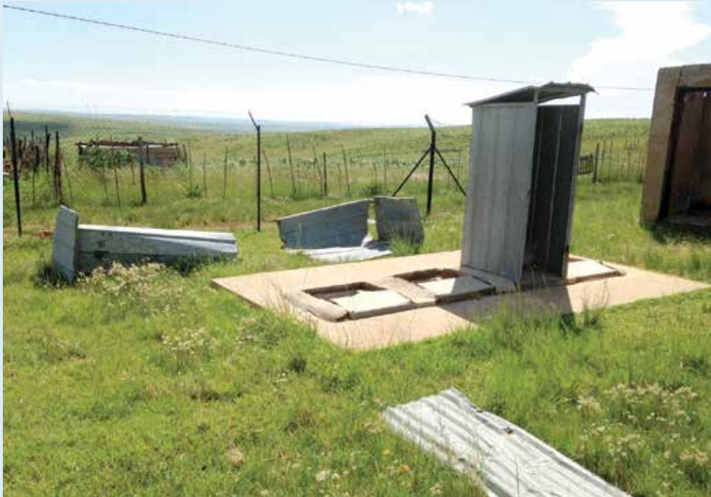
Adequate construction and maintenance of toilet facilities is a significant issue at many schools.
