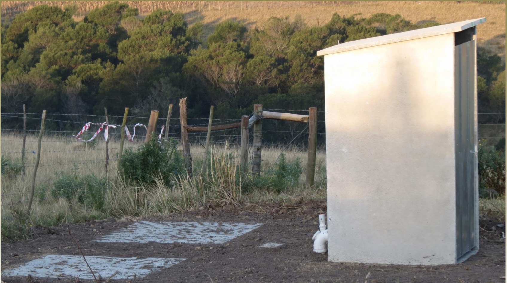
Pour Flush toilet at Jerseyvale, near Stutterheim, Eastern Cape
