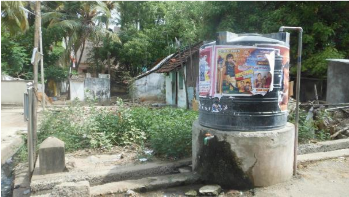
Plate 3-2: Mini Power Pumps for Non-potable Water in Pammal
