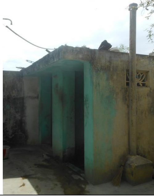
Plate 3-5: Shared Toilet in Pammal
