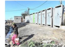
Communal toilets are seen at an informal settlement in Cape Town. The writer says authorities are faced with the challenges of providing hygienic human waste disposal fast enough to accommodate thousands migrating to the city. Photo: Courtney Africa
