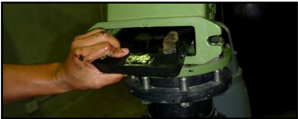
Figure 23: When assessing why the discharge pump was not working, pump station operators realised that the vessel’s non-return valve was upside down and had somehow collected stones (Taing, 30 March 2011). The operators conjectured that the ‘pipes’ team might have unintentionally inserted the valve upside down when attempting to address potential vacuum station problems without the ‘pumps’ team.
