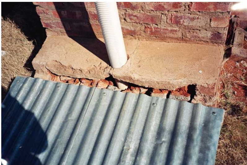
Figure 6.11: Examples of poor practice (2): These vaults are not sealed against ingress of flies, rodents, snakes, rainwater, etc (Photographs: CSIR)
