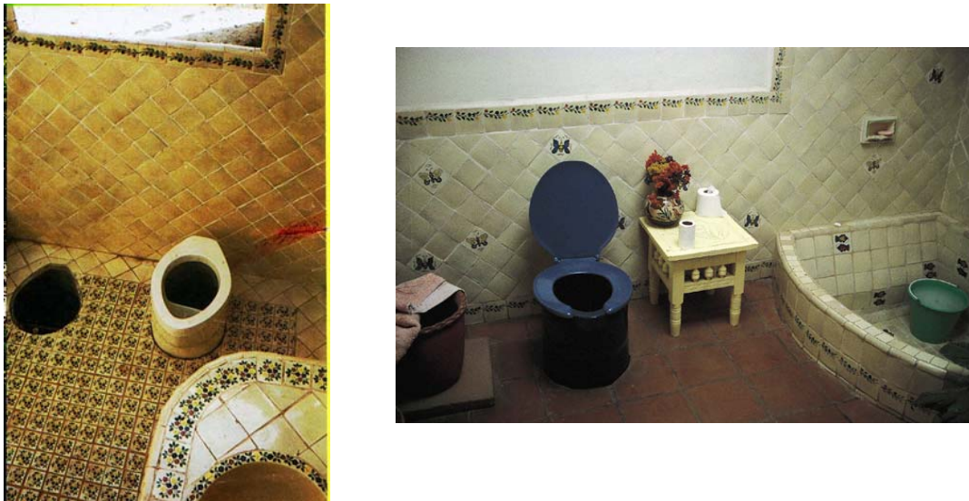
Figure 2.9: The Mexican version of the Vietnamese double-vault toilet, installed in the bathrooms of modern houses in the city of Cuernavaca. The toilets have movable urine-diversion pedestals. The processing chambers below the bathroom floor are accessible from outside the house (César Añorve, CITA, A.C., Mexico)
