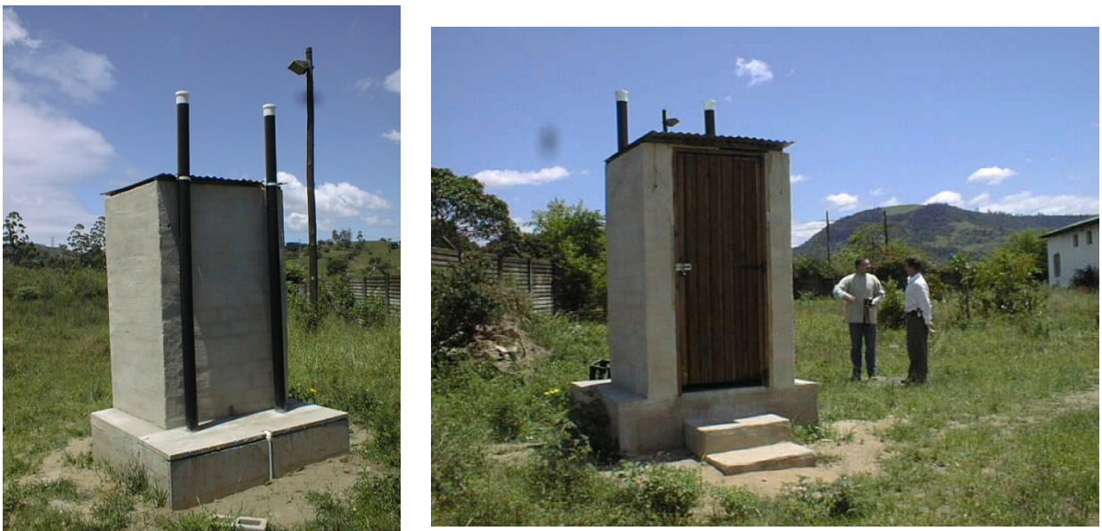
Figure 5.1: Typical double vault UD toilets built in the eThekweni municipal area. Vaults similar to these, without the superstructures, were constructed for the experimental work at NWWTW
