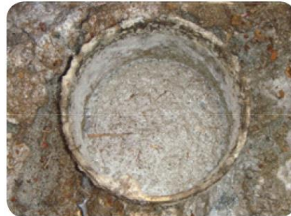
Solidified layer of sludge in de-sludging pipe
