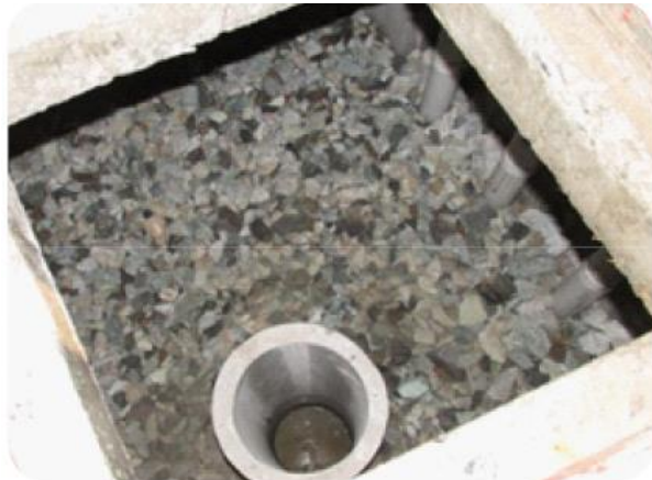
Sludge in the de-sludging pipe
