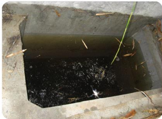
Debris in collection tank
