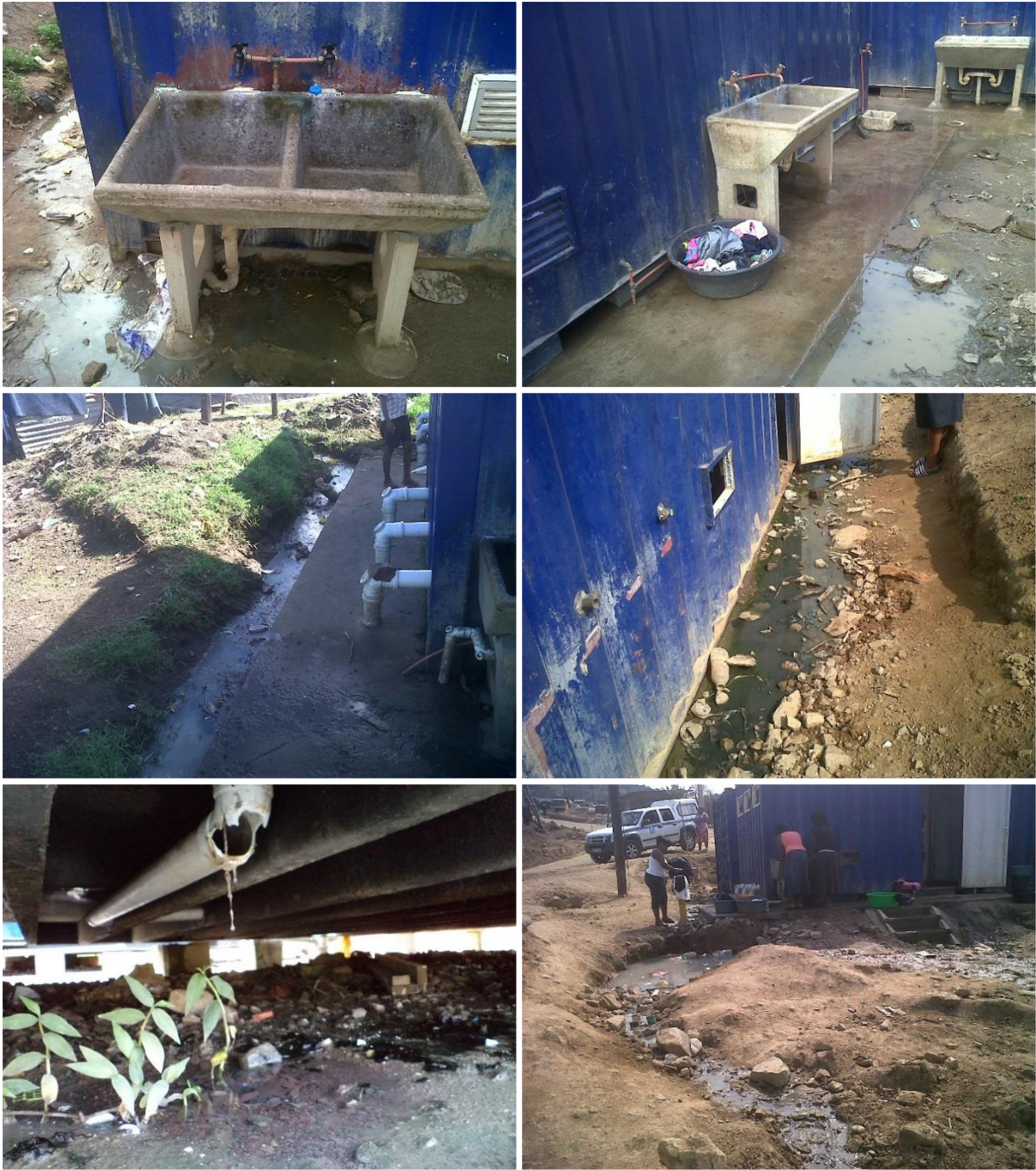
Figure 2: Poor drainage externally in the CABs
