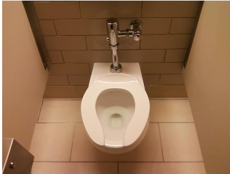
Figure 3: Typical public toilet using a demand flush at the Aquaduct Racetrack Casino (see Chapter 9)
