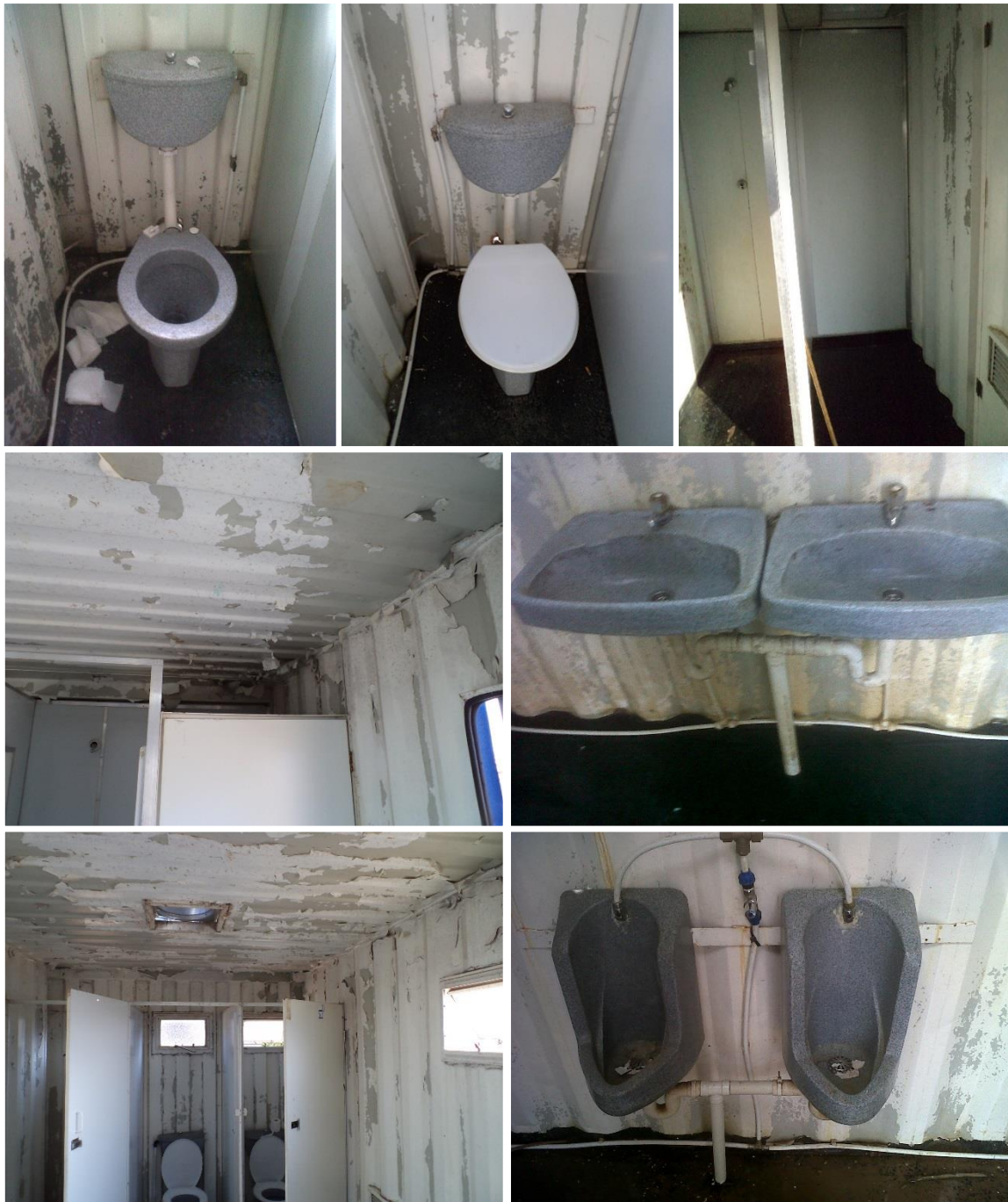
Figure 14: The paint chipping off on the inside of a CAB
