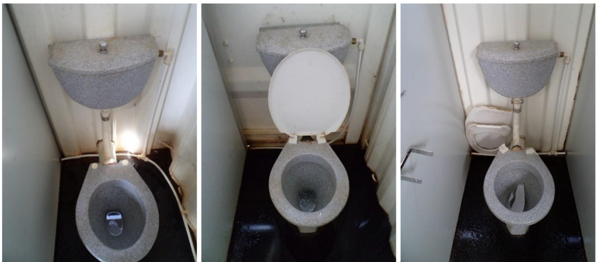
Figure 23: Missing and broken toilet seats (August 2012)
