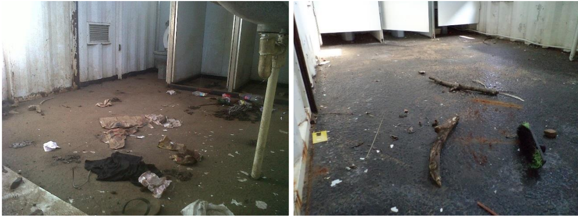
Figure 9: The vandalism associated with missing air vents in the CABs
