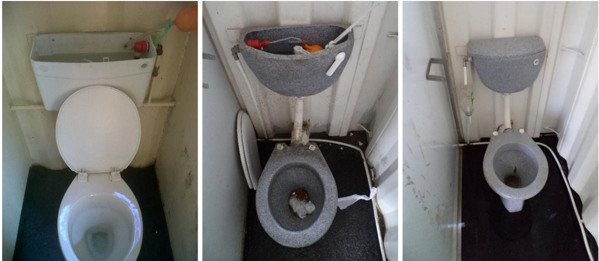
Figure 22: The broken flush mechanism from the CAB toilet cisterns (August 2012)
