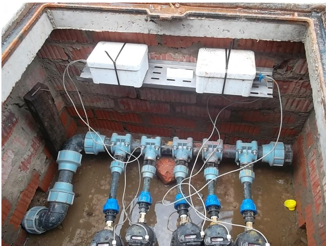
Figure 7: The internal configuration of the data logging equipment at one of the male CABs in Frasers. The water meters are shown at the bottom of the figure, and the data loggers are elevated in order to ensure that they do not suffer water damage during rain or due to leaks (Mohan 2012).
