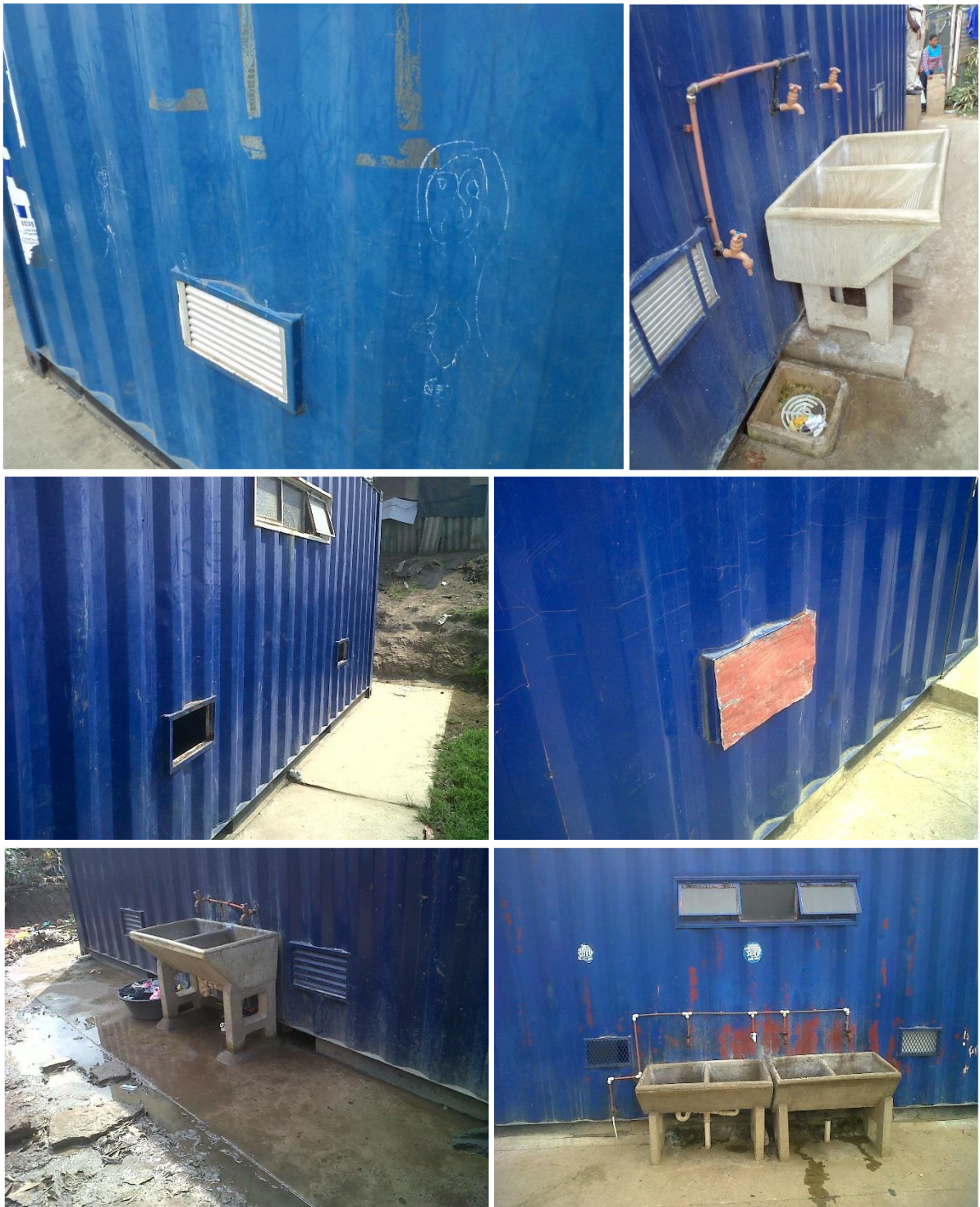
Figure 8: Types of air vents found in the CAB facilities
