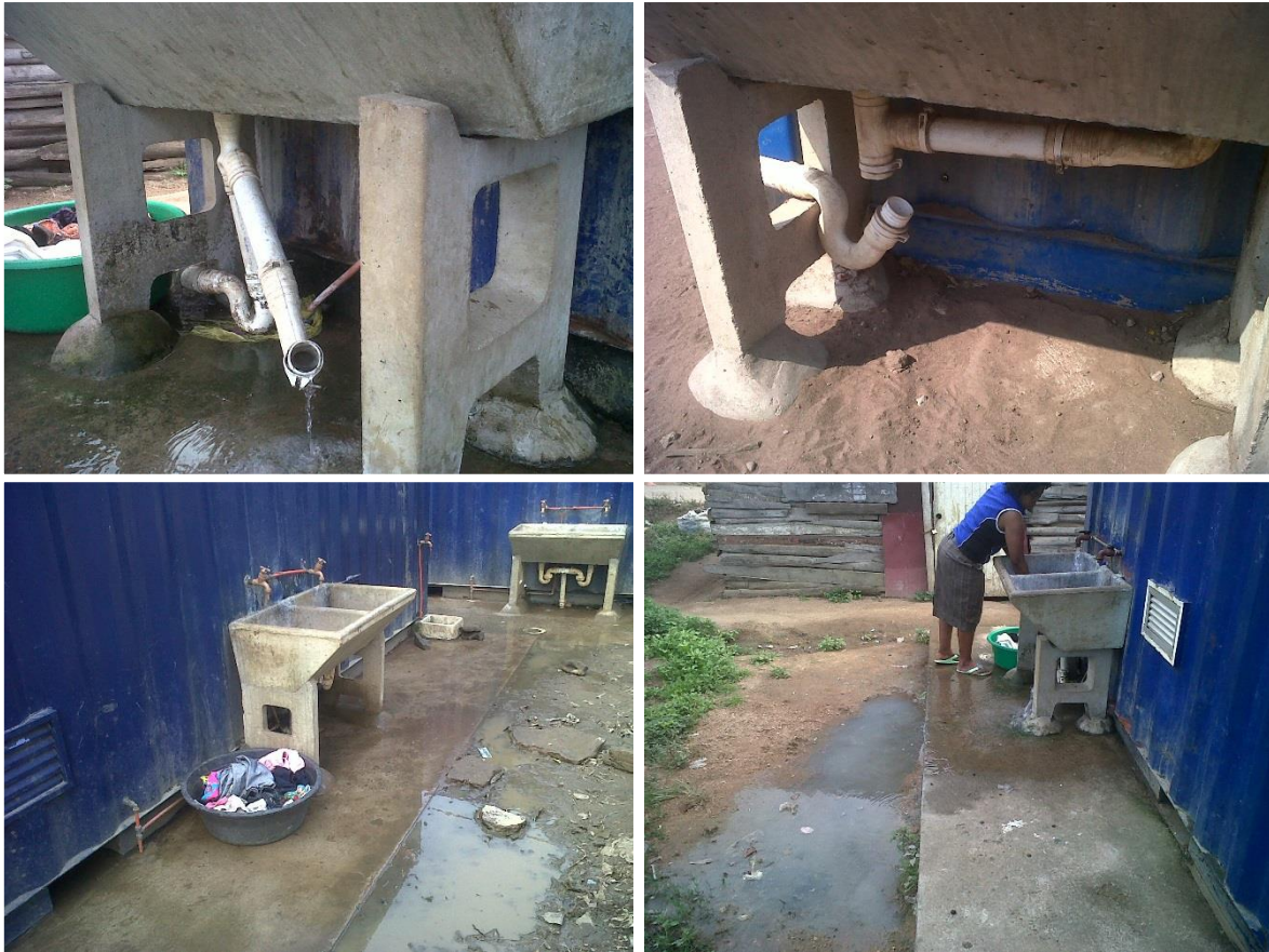
Figure 28: The problems associated with the wastewater discharged from the laundry facilities The top photos show how the discharge pipes from the laundry facilities have loosened from the basin and discharges water directly into the surrounding environment. The facility in the top left photo is dry due to the water being turned off at the CAB facility due to other broken sanitary fittings. The bottom photos indicate the greywater discharges into the environment due to poor drainage of the laundry facilities. Although not directly investigated, this poor drainage could also be due to the users performing washing in buckets and discharging the wastewater next to the basins.
