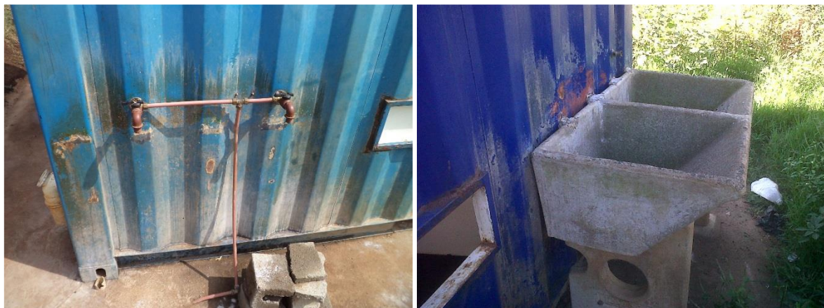
Figure 27: The problems associated with the laundry facility structures
