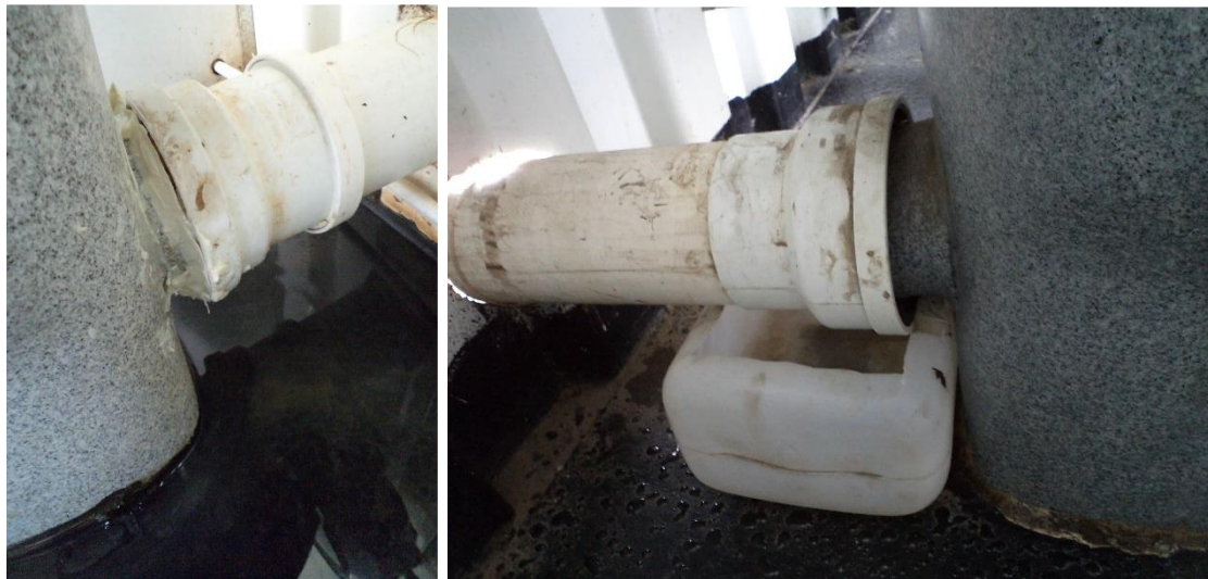
Figure 21: Leaks from the toilet discharge pipe
