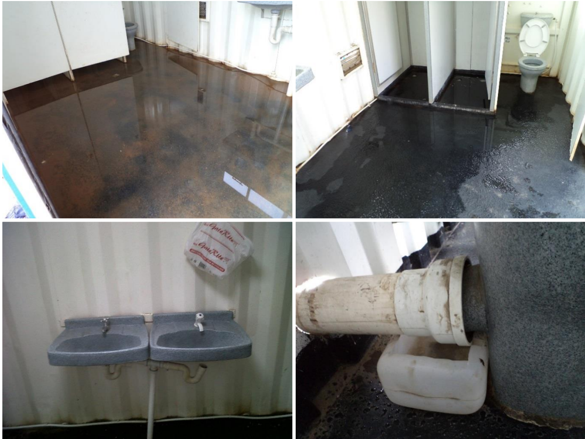
Figure 3: Poor drainage internally in the CABs
