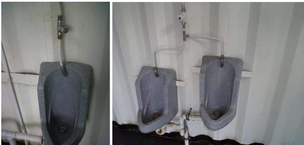
Figure 4: Typical urinal configuration in the CABs in eThekweni (August 2012)
