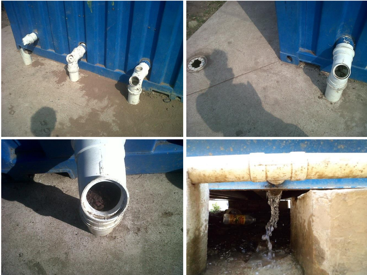
Figure 32: Vandalism of the discharge pipes
