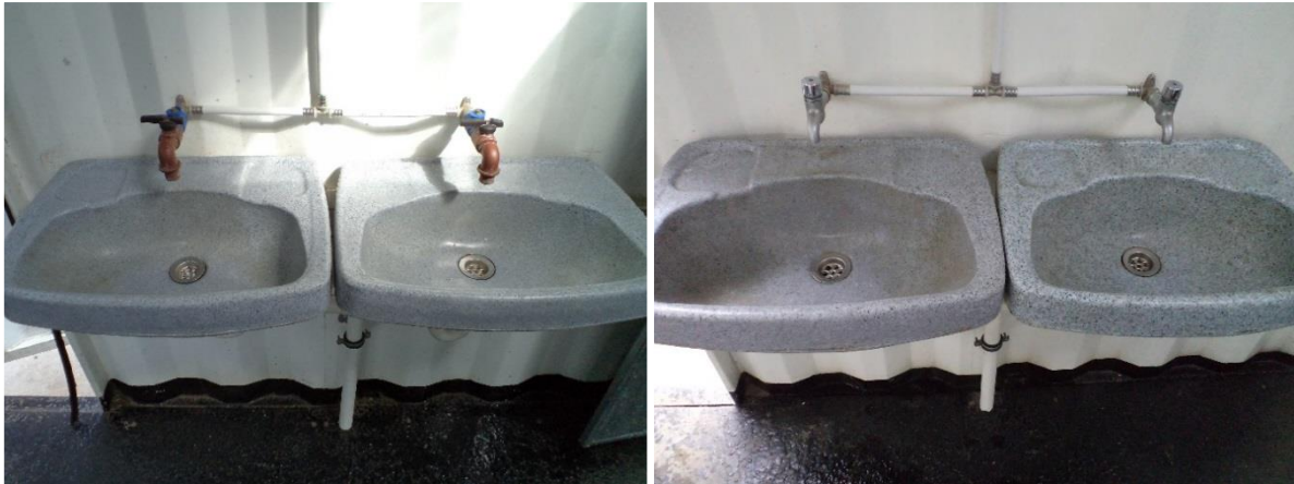
Figure 20: The wash hand basin taps fasted to the walls of the CAB
