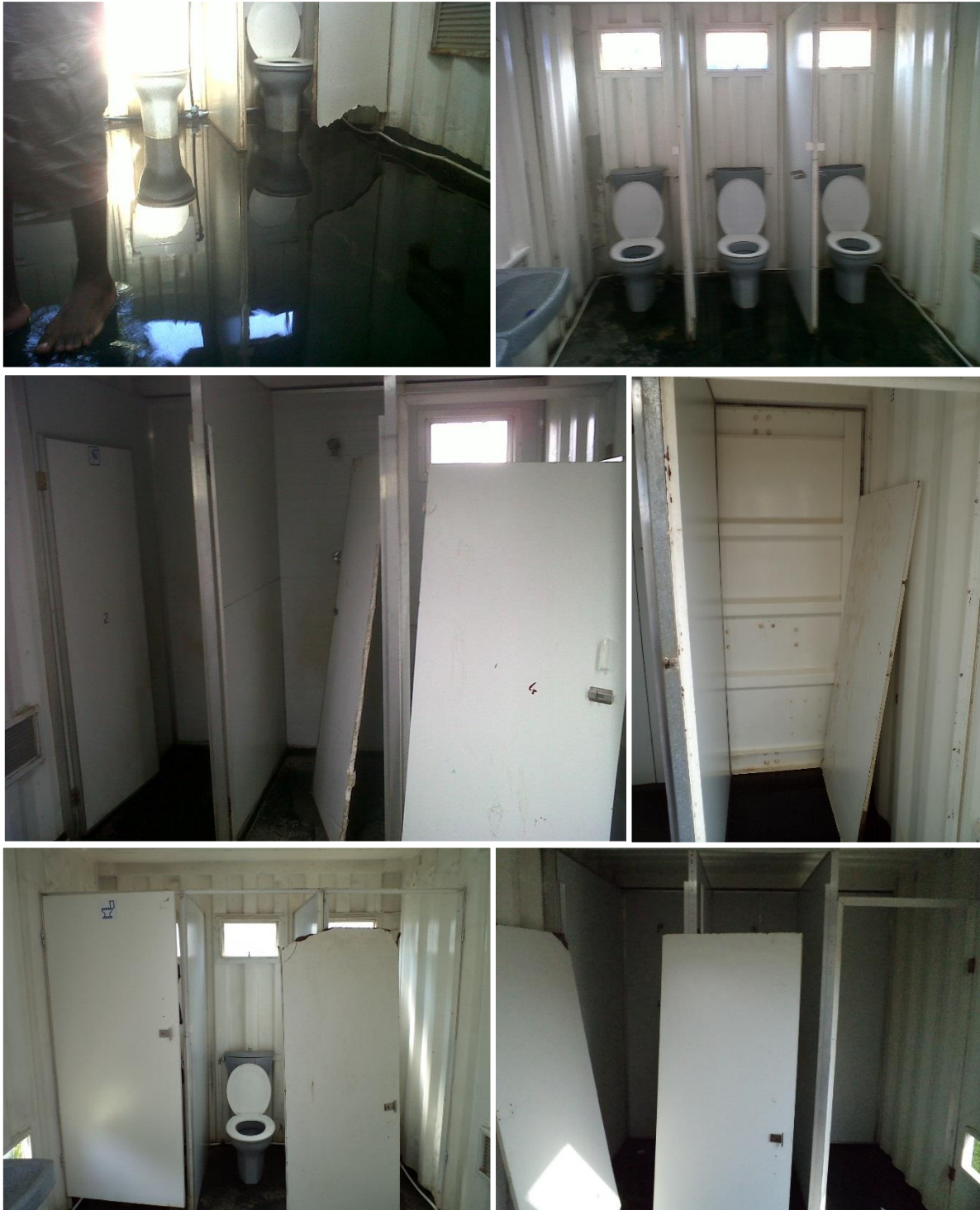
Figure 11: Photographic evidence of the broken and missing cubicle doors
